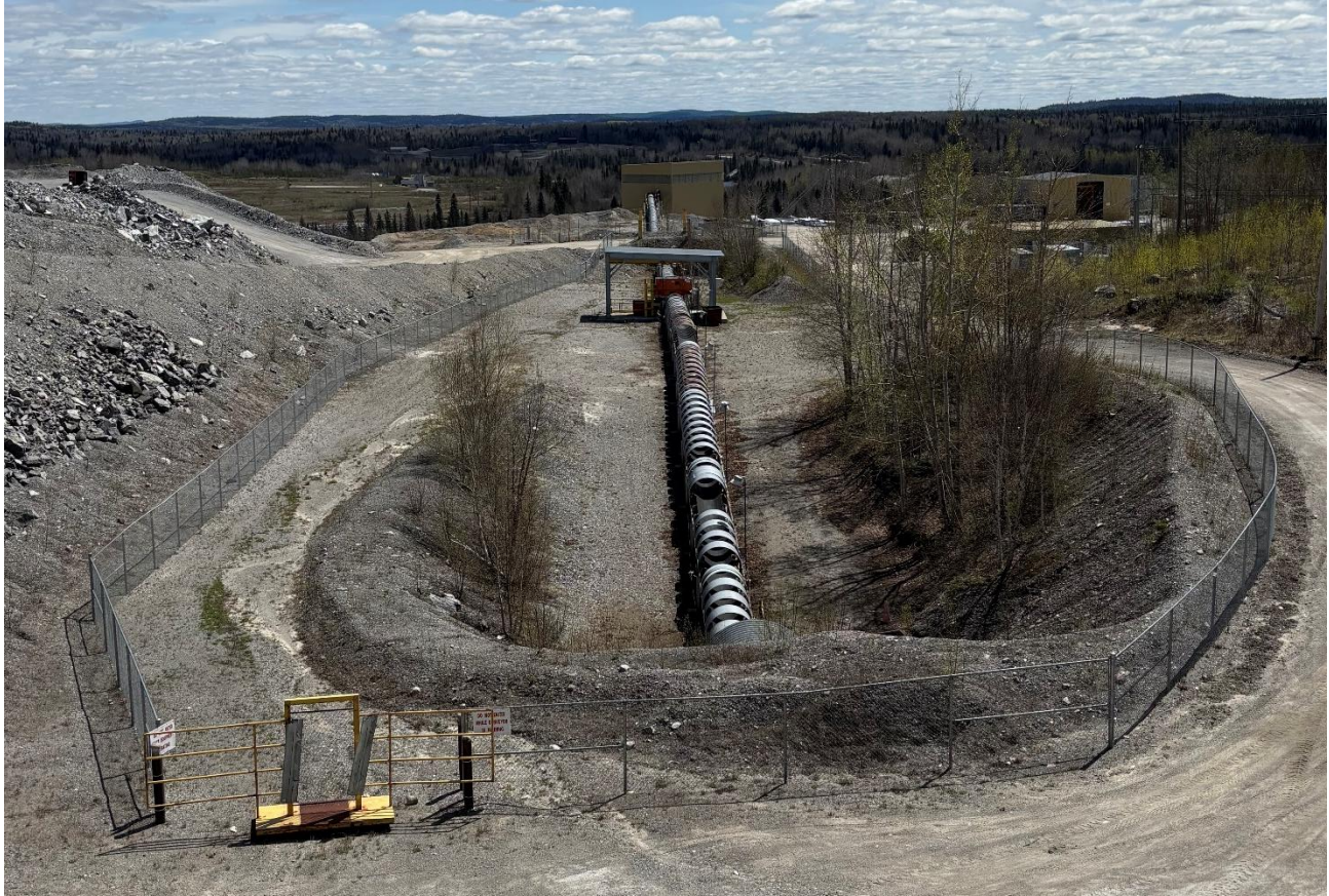
Figure 18-7: Conveyor #10, from the Crusher to the Screen Building
