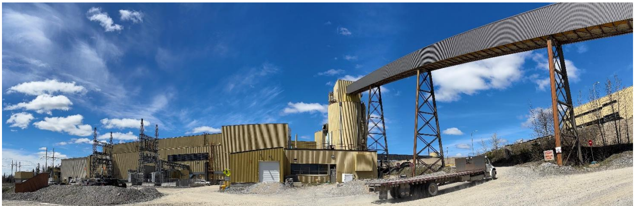
Figure 18-11: Conveyor #3 to Coarse Ore Bins at the Mill
