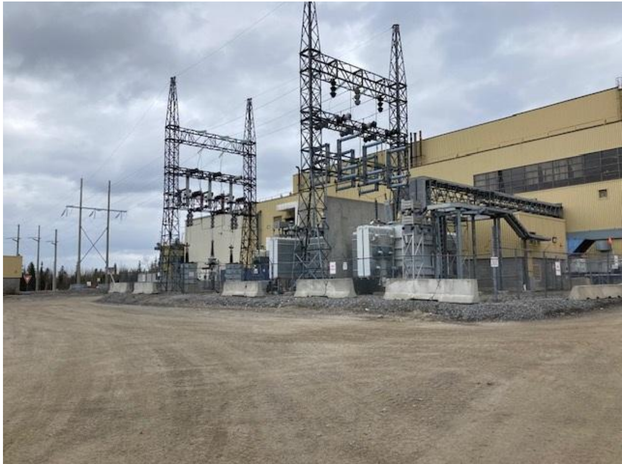
Figure 18-5: Hemlo Substation and Transformers
