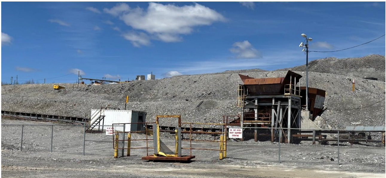
Figure 18-9: Conveyor #19 Loading Hopper
